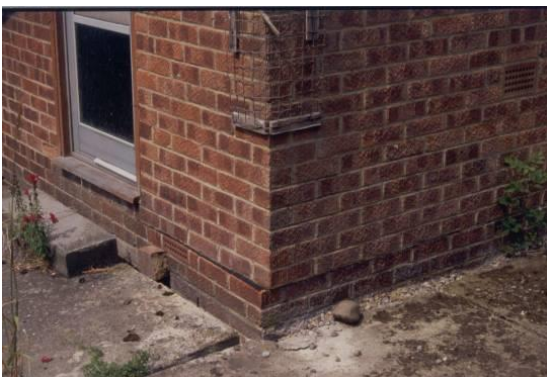
Movement along damp-proof course
