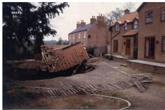
Collapse of detached garage
